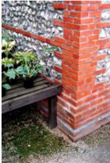
Figure 34: A corner of the building. Interlock of brick and flint throughout the building.
