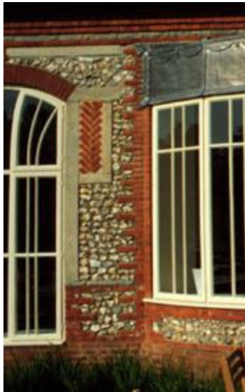
Figure 36: Lack of Deep Interlock on south facade where great windows meet curved window. The respective systems start and stop abruptly and there is little interlock. The interlocked brick and flint help a little but seems weak relative to the size of the adjacent 'centers', and it does not engage the brick and concrete panel system to the right of the Dining Hall window (at left).
