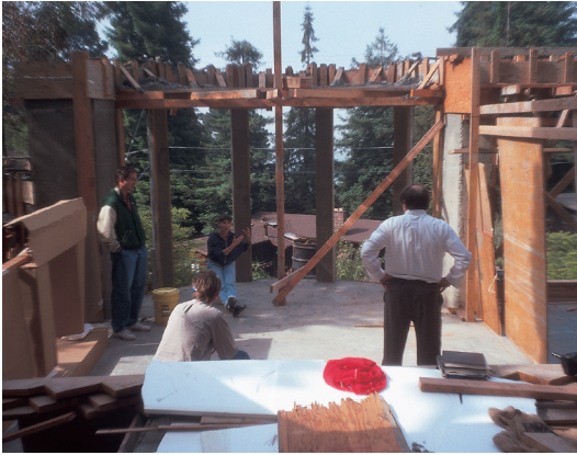
Upham house: settling positions of columns, to form the bays, and window openings of the living room bay window.
