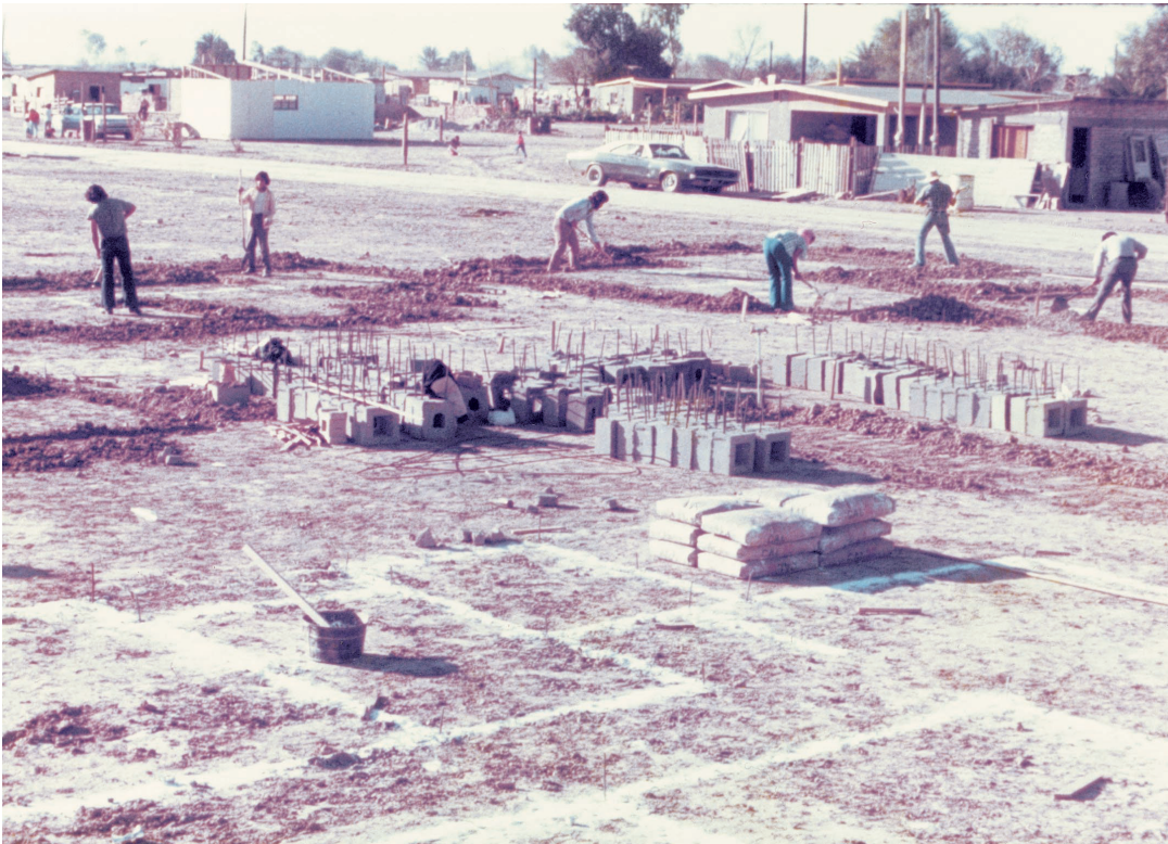
Forming centers in the early stages of a house-building process in Mexico. From the very start, the emphasis is on step-by-step adaptation: design and construction are integrated. Christopher Alexander, Julio Martinez, Howard Davis, and others, Mexicali, 1976.
