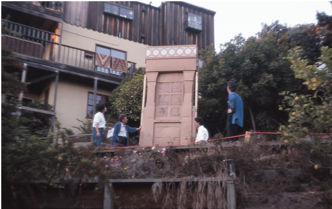
Cardboard mockup of wall construction. This mockup was very detailed, full size, and allowed us to check the offset between one plane and another to the nearest half inch and quarter inch
