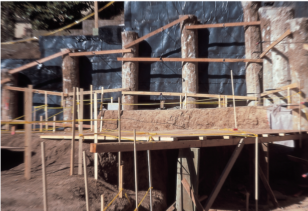
The piers exposed after drilling and pouring, and ready for forming the foundation and retaining wall between the piers
