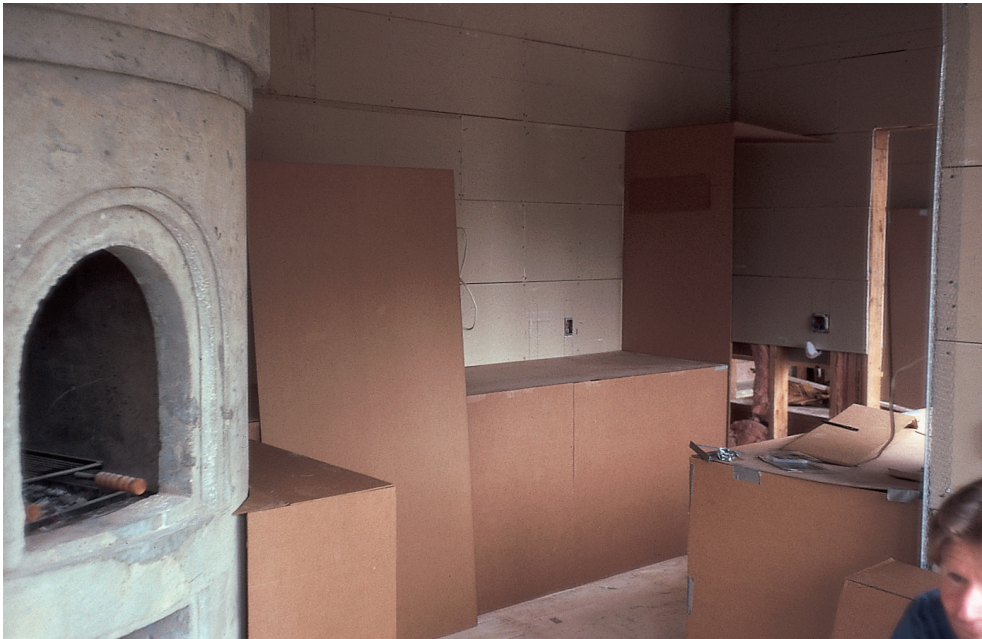
The kitchen mocked up in its entirety in cardboard, so we could see just how to make the kitchen fireplace. The idea of a cylinder had already occurred to me from seeing the room shape and recognizing its two lines of sight. Now we had to make the cylinder work, and to do that we had to have the full three-dimensional configuration, as it was going to be. We had to make many many versions before it all sat right.
