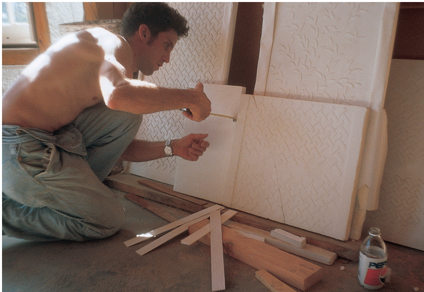
Randy checking widths and details of the edge band on the plaster panels. On these panels, it turned out that a difference among one-eighth, one-quarter, and three-eighths of an inch was of tremendous significance.
