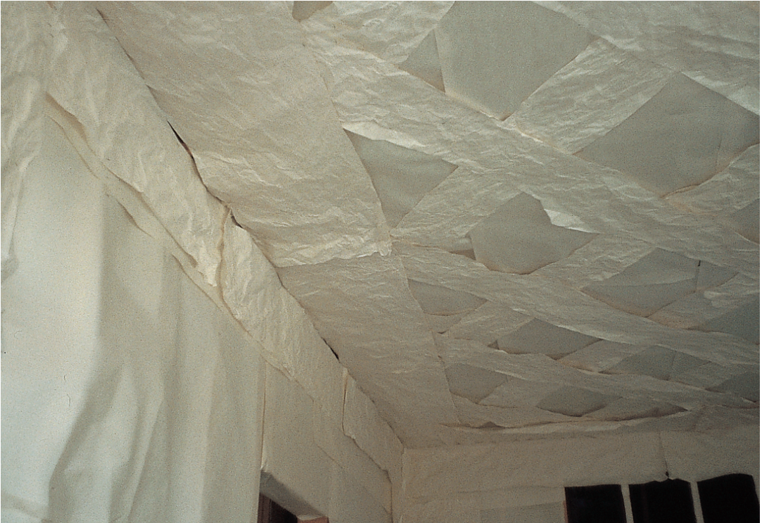
Mockup in paper to test the overall pattern of the plaster panels on the ceiling. This part concentrates on the edge, where the width of the panels had to be chosen very carefully, to get a proper harmony.
