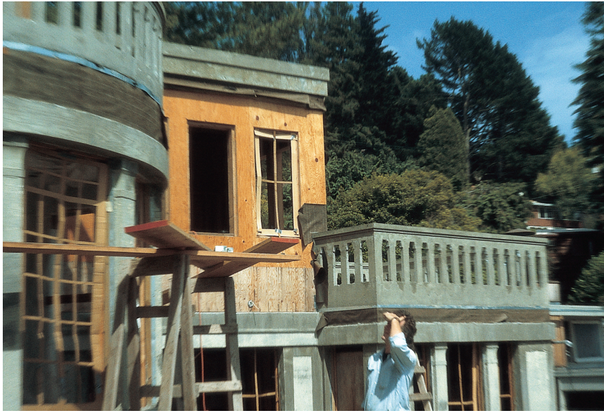
Before ordering windows, we made cardboard mockups of the glazing bar and pane layout in every window in the house, and examined them from inside for their effect on the room, and from outside for their effect on the street
