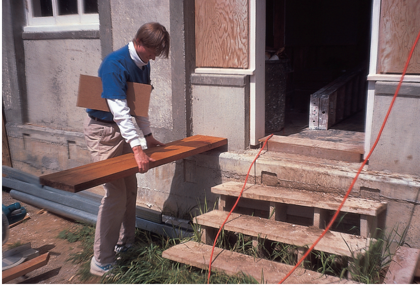
Using a simple board to judge the height, width, and length of a concrete parapet which was to be built on both sides of the concrete front door steps
