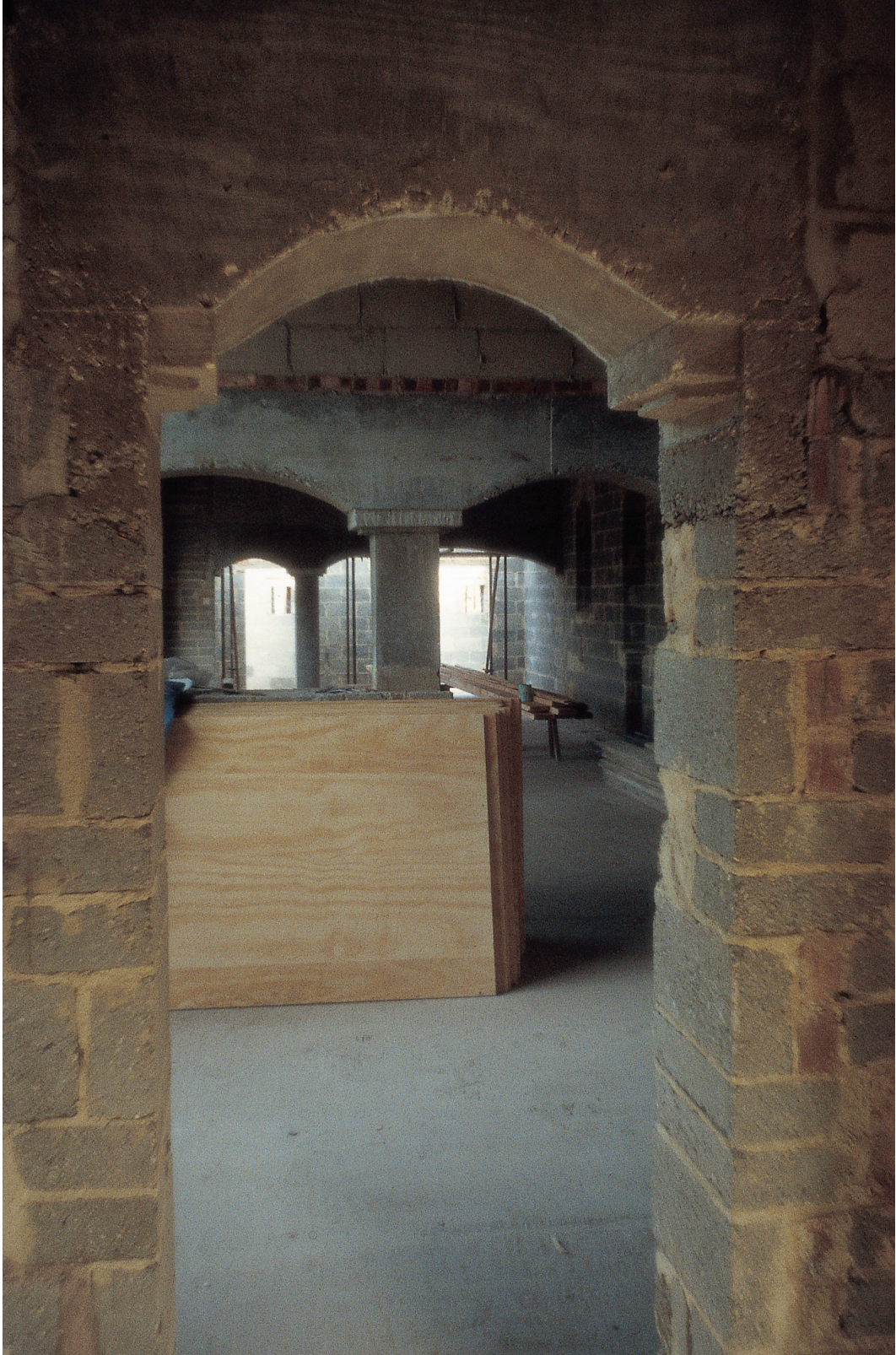
One of the openings, as it developed in rough block and concrete
