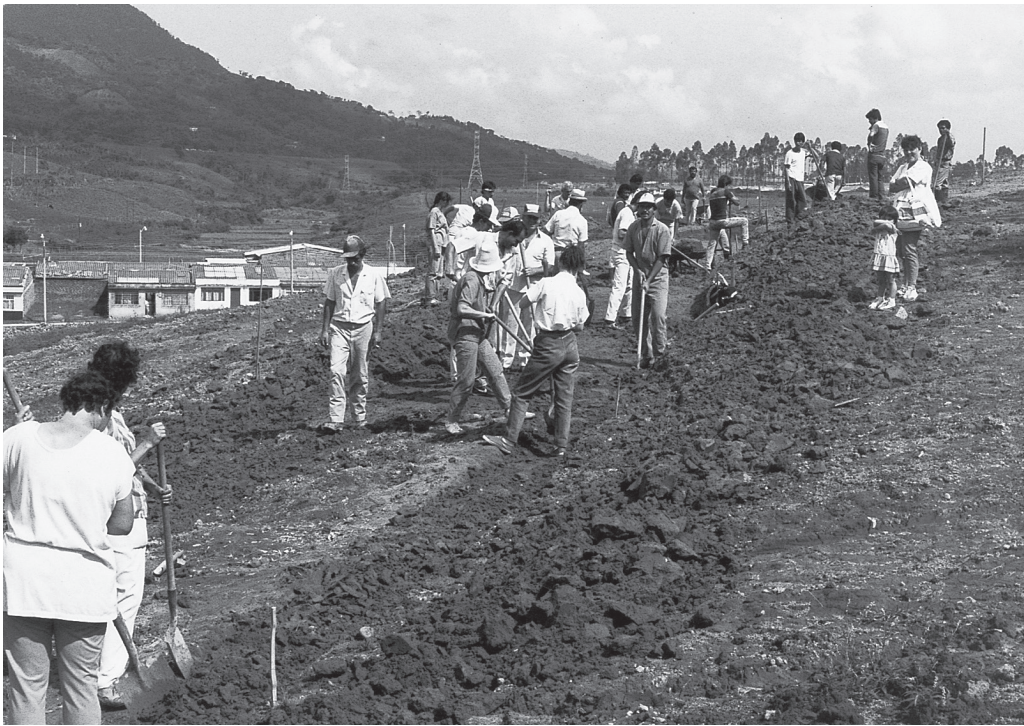
Starting work on the main sewage trenching, Santa Rosa de Cabal, Colombia, 1991.
