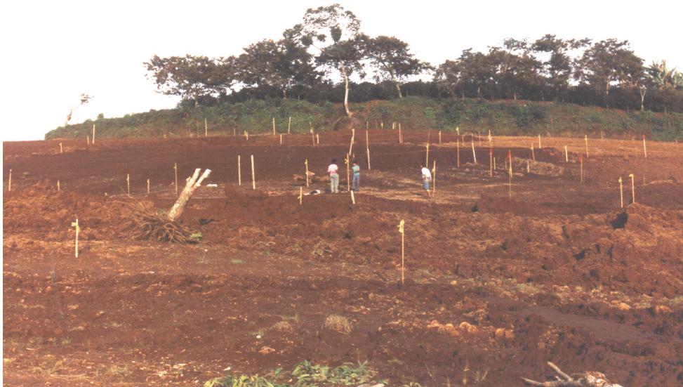
The first step taken in designing a new neighborhood. Santa Rosa de Cabal, Colombia. Neighborhood of seventy-six houses, built by families. Construyamos and CES, Christopher Alexander, Ingrid King, Kleoniki Tsoutropoulou, Fanta Lawrence, Seth Wachtel, Jeannie Radcliffe, and others, 1990.
