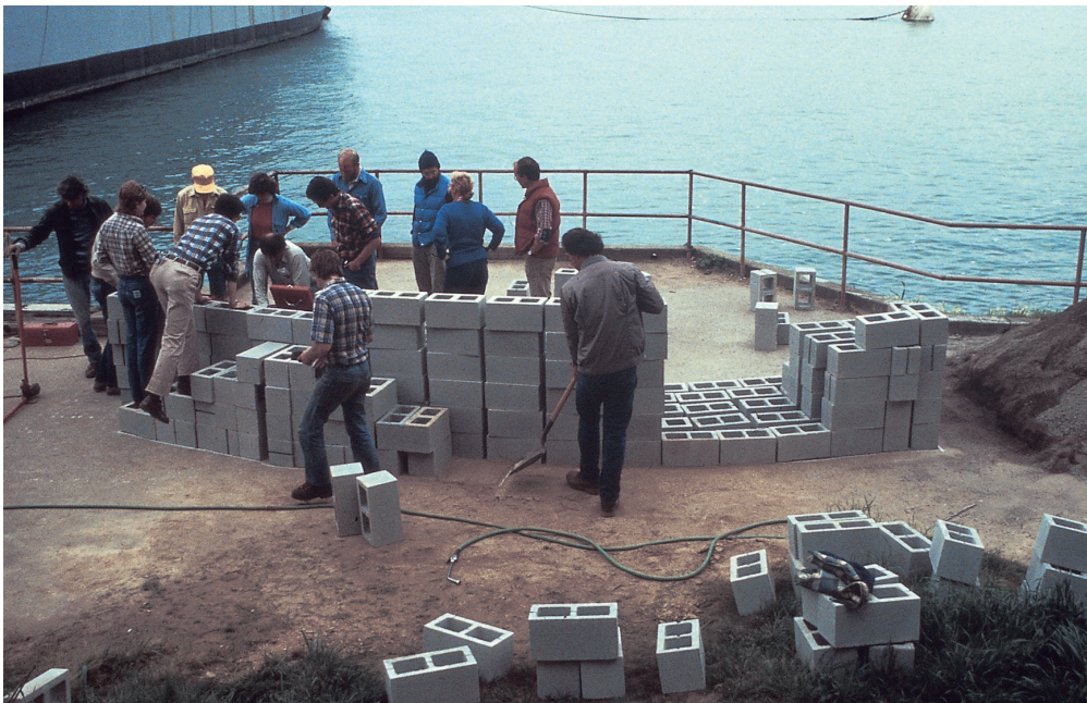
Fort Mason Bench, San Francisco, Placing dry-stacked concrete blocks to get the right arrangement of the bench. Christopher Alexander and students, 1988.
