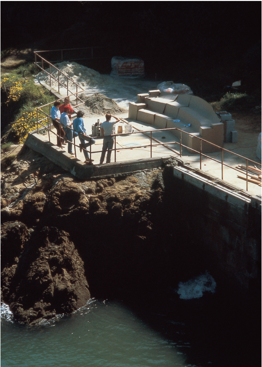
Last look at mockups, deciding the right shape and size and height, before starting on the work of building the actual bench. Fort Mason, San Francisco, 1985.
