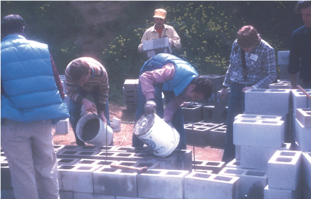
After the mockup showed us where to place the bench, we used the same blocks to build the armature. Here, people are beginning to pour concrete into the first course of blocks.
