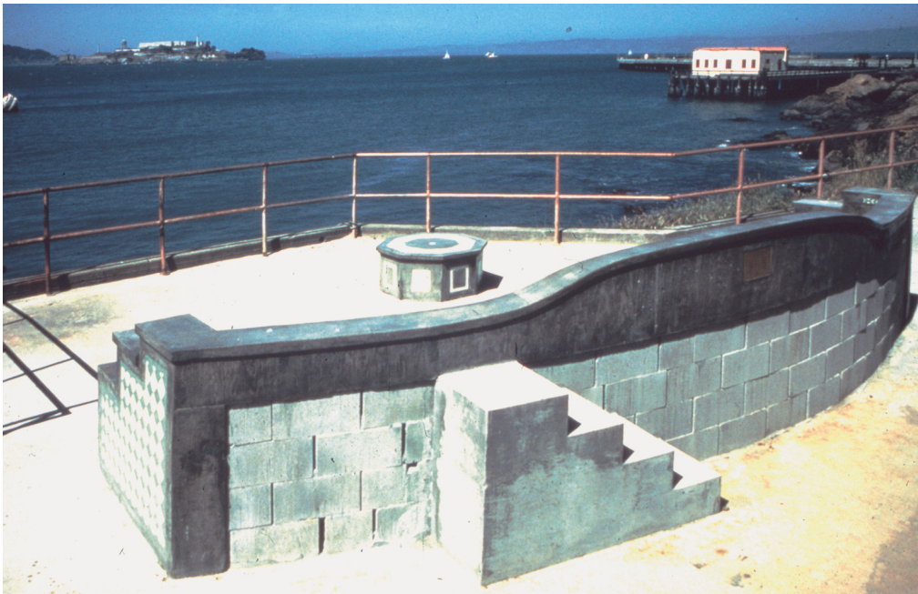
The beautiful forms that arose from the process of placing dry-stacked concrete blocks to get the right arrangement of the bench. The steps were put in spontaneously, late in the game, to give access to the upper tier of seats.
