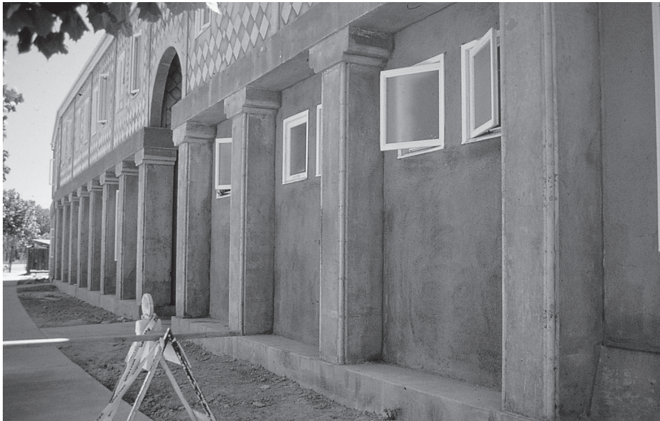
Wall surface of the Julian Street Inn, a continuous waterproof surface of cast concrete columns and heavy frame walls, forming centers that are latent in the structure of the undifferentiated plane and of the bays.
