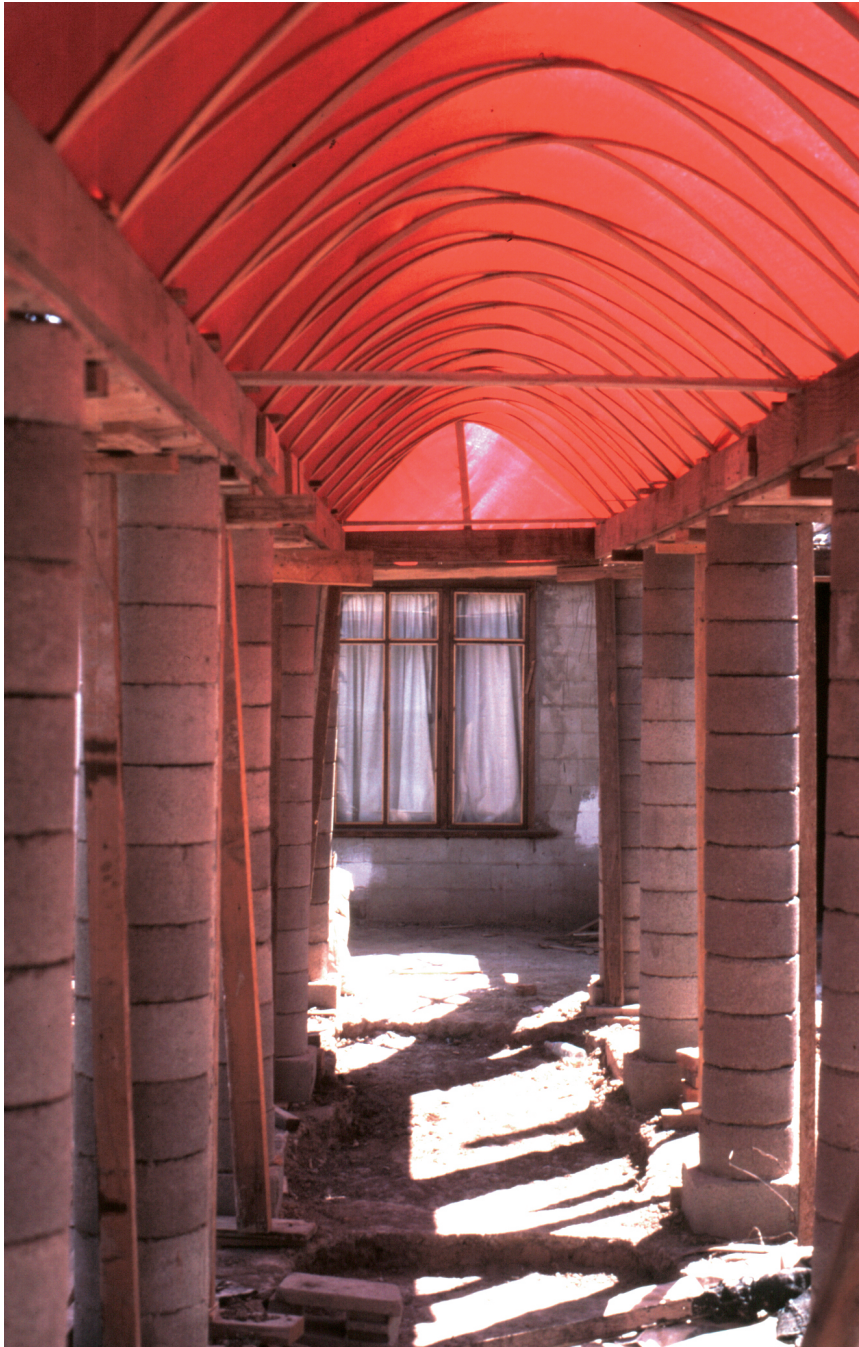
Columns with substance, made from specially manufactured cylindrical blocks of soil-cement, cast and pressed on our own modified Rosa-Cometa block-making machine, Mexicali. Christopher Alexander, Julio Martinez, Donald Corner and Howard Davis, 1976.
