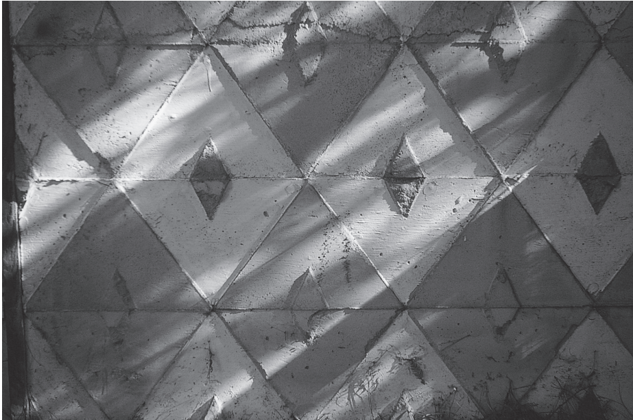
Ornamented concrete wall panel, cast, with layers of diamonds cast into the panel in the vertical position. Christopher Alexander, 1986.
