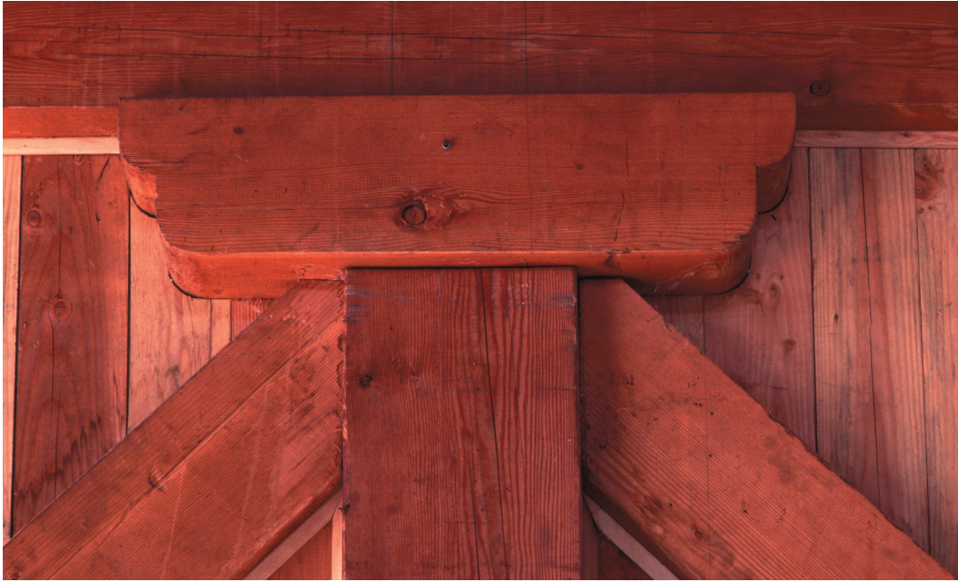
Capital where braces, beam and column meet, Martinez Carpentry Shop, Christopher Alexander, Gary Black, Seth Wachtel, 1986.
