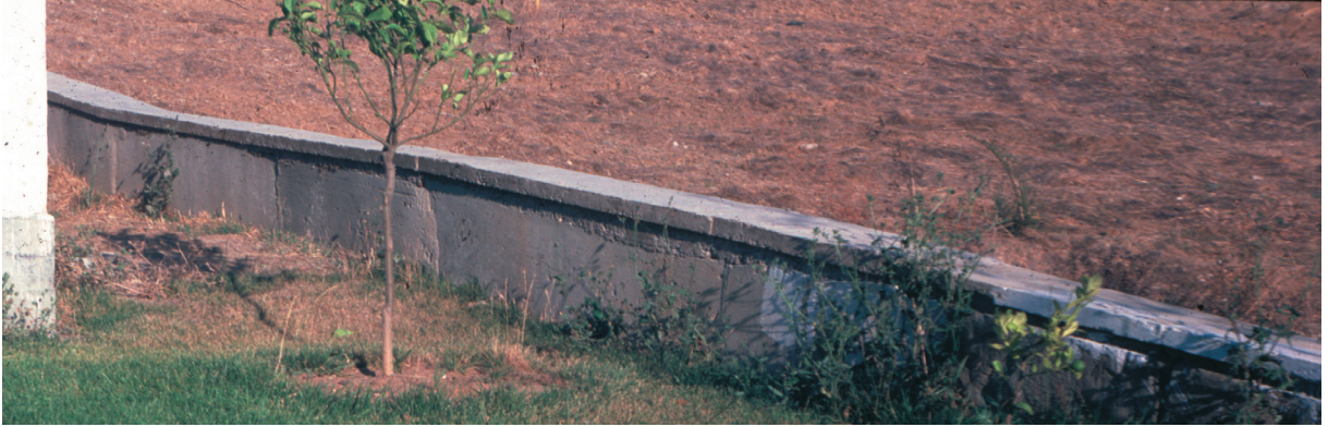
Very robust garden wall made from old hardened-up cement sacks, with a poured concrete cap; the surface of the bags was shot in low-budget shotcrete. See discussion in Book 4, pages 130–31.
