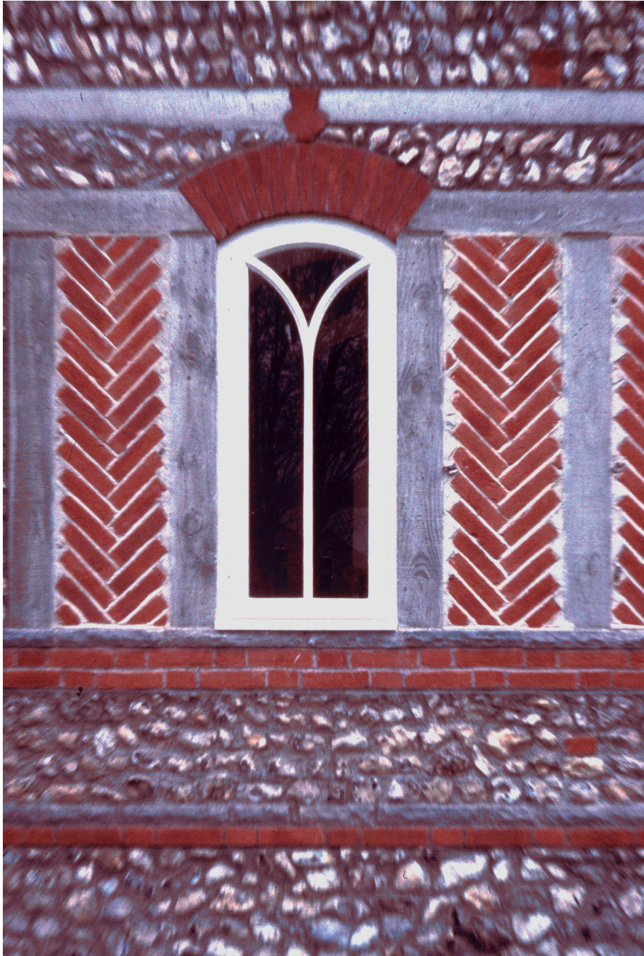
This wall segment, part of the construction of the West Dean Visitor's Centre, West Sussex, England, shows a fully integrated masonry structure in which brick, stone, concrete, tile, and wood cooperate structurally, and in a way that permits individual shaping and sizing of all the elements without compromising structural integrity. 1996.
