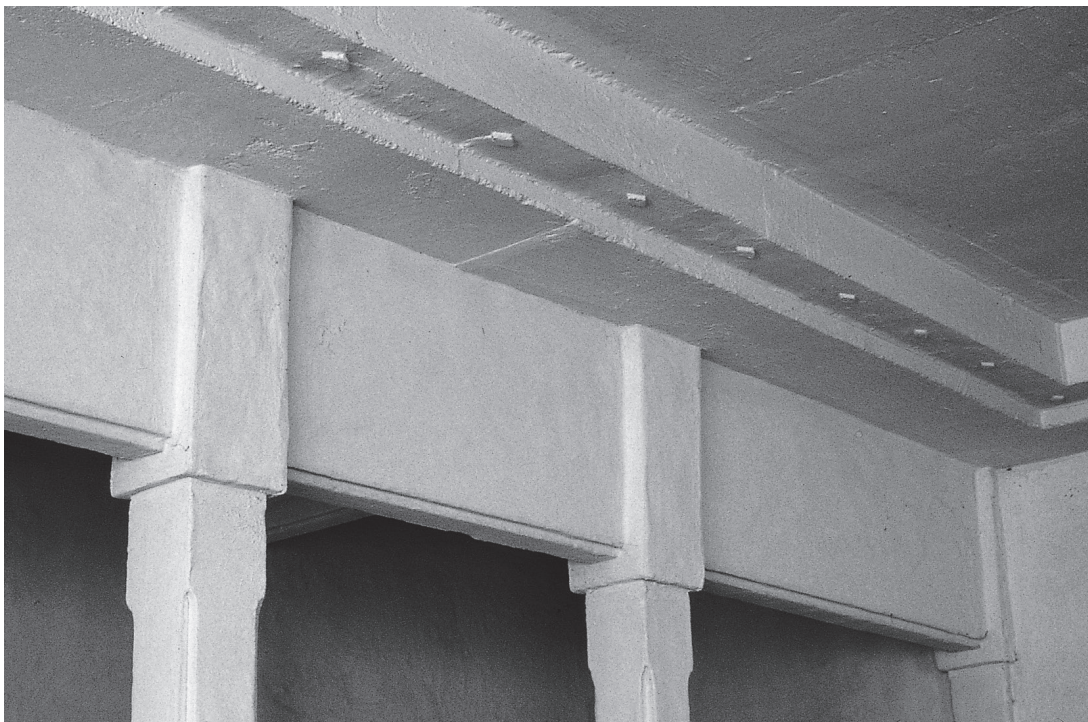
In the shaping of the beam, column, column capital, we see the beginnings of powerful centers being formed — in this case with the cheapest formwork and with a very crude concrete shoot that nevertheless goes a long way to bring this inert piece of concrete to life. Martinez House, California.
