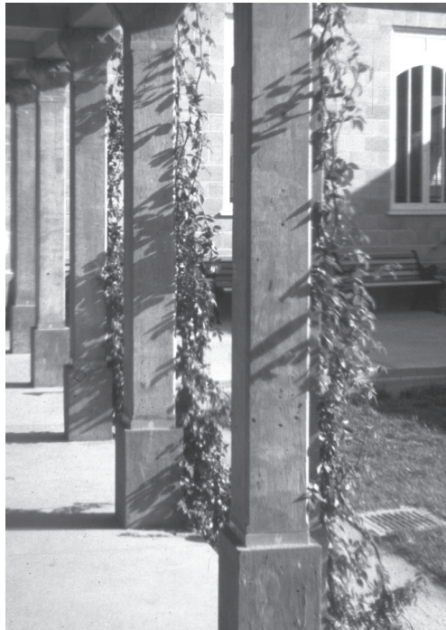
Shaped cast bases on the columns from the Julian Street Inn, San Jose, precast and formed in our Martinez yard.
