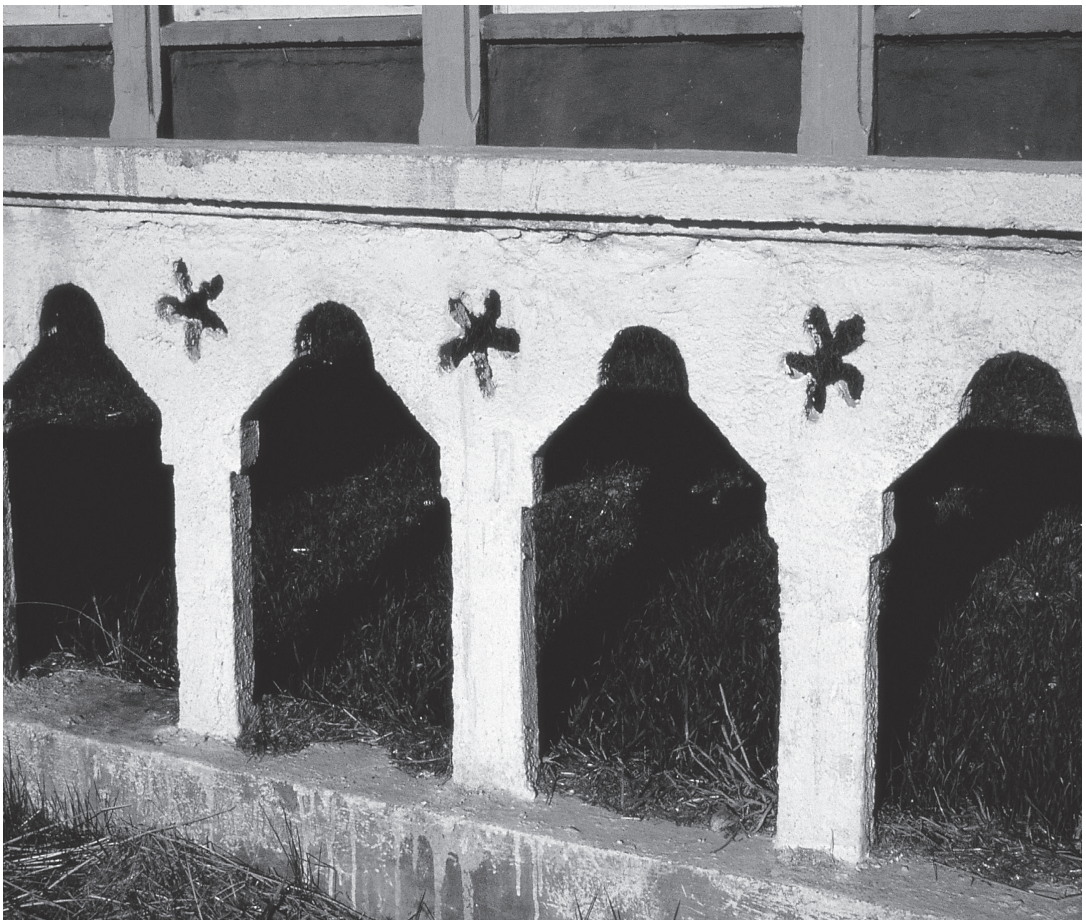
Balustrade in which arches, columns, and flowers are formed with cheap foam inserts, pinned onto a sheetrock backing, and shot with gunite. Christopher Alexander and David Dacus, 1980.
