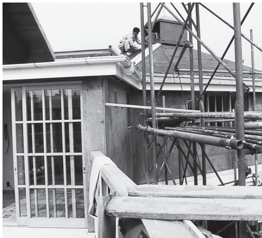
Fifth-floor penthouse, Emoto building, Tokyo, while design and construction were still going forward together.
