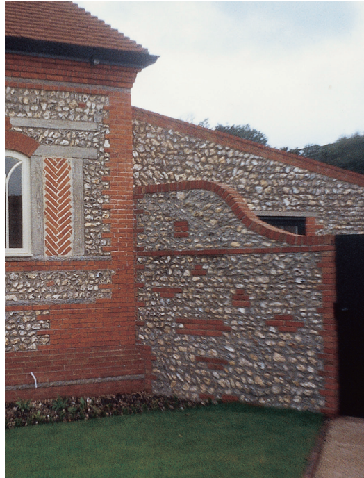
Because the window is so close to the corner, the brickwork goes differently here.
