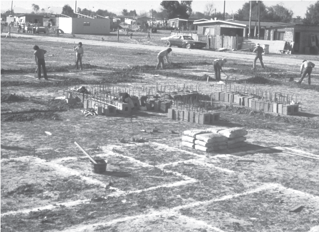
Laying out houses in Mexicali. It is “making” from the very start; design and construction are integrated. Mexicali, 1976.
