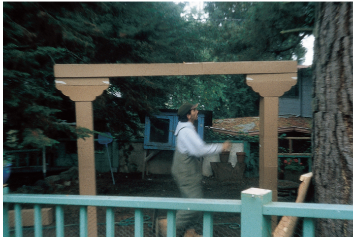
Third try, another version of the same capital. This time we got the proportion, size, and spacing just about right. This is what we then built in the actual project. See photograph below.
