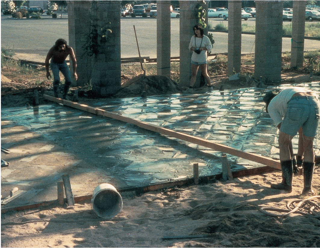
Working the slab of our 6000-square-foot floor in the Fresno Farmer's Market. Here we dropped prefabricated indented polygons of blue concrete, half an inch thick, into the wet slab and made them integral with the whole. Each took its position according to the wetness of the material, the time it was worked, and the setting of the concrete. The resulting uneven surface, like a fish's scales, shimmers in the sun.
