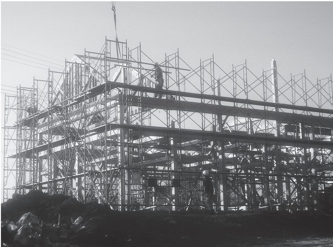
Heavy carpentry work on a fairly large building, one of ours, under construction in Japan.
