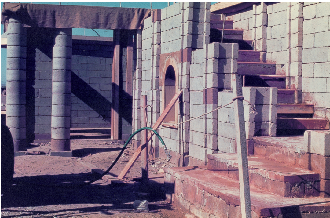
Dry stacked blockwork when walls are almost complete and have had some cells filled.
