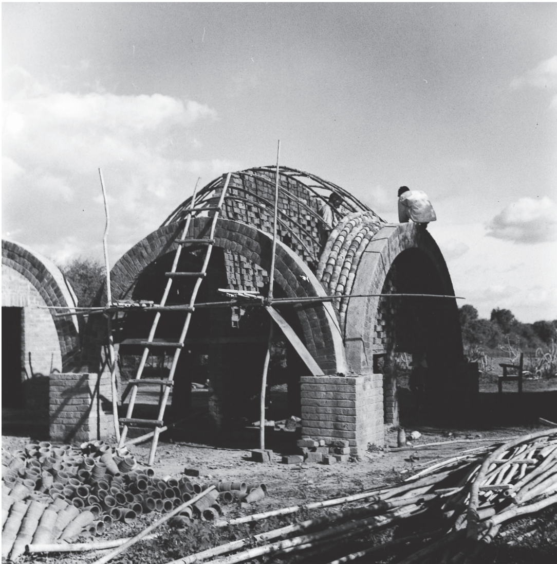
Formation of domes in a way that could be made using tiles made by the village potter first forming guna-tile ribs in the dome, then plastering them lightly to form the complete dome.
