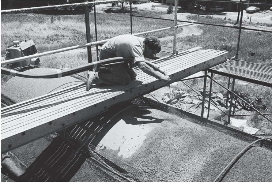
Shooting gunite over forms to make the ceiling vault and roof of the workshop. I spent hours on that bridge shooting a fine stream of material to shape the outer vault surfaces.
