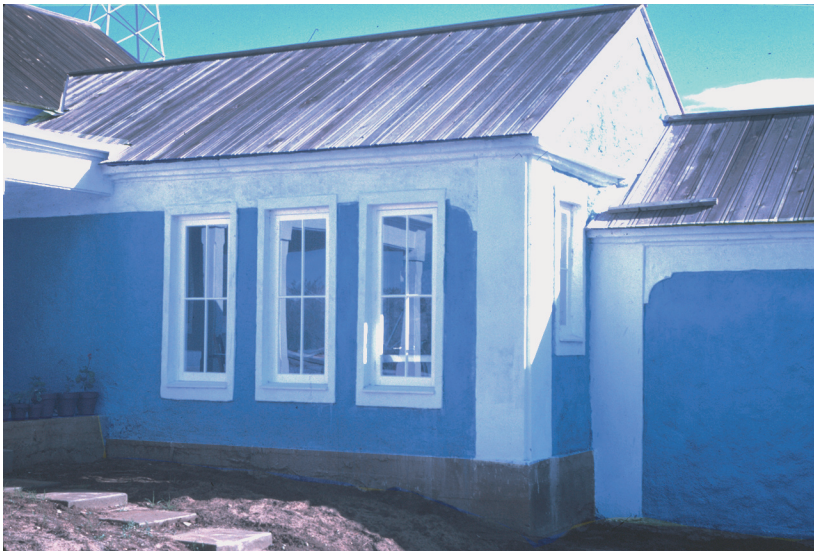
Martinez house from the side, after the shoot, and after roof surface and windows have been installed
