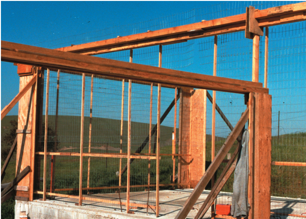
Light weight, low-cost guidework before shooting the Martinez house in gunite. Note the extreme lightness of the guidework, as it is first put up, which allows easy creation of beautiful shape and proportion.
