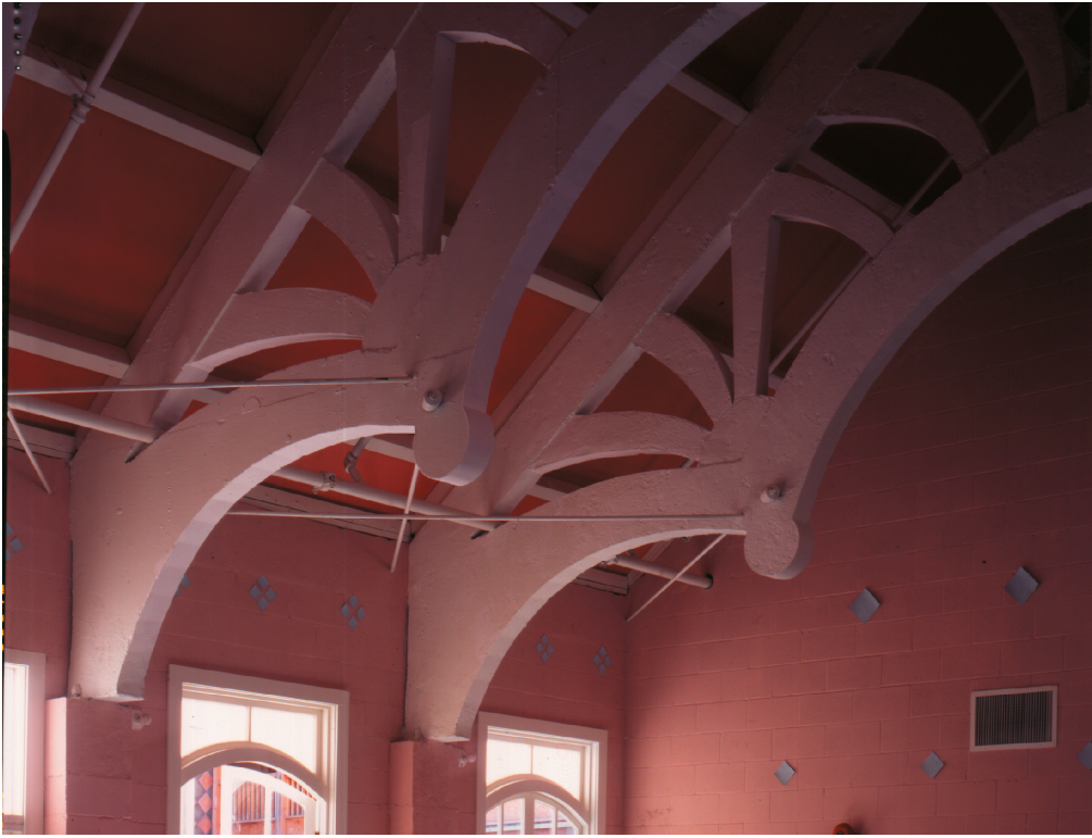
Two of the series of lacework concrete trusses we shot in the San Jose Homeless Shelter. Christopher Alexander, Gary Black, Carl Lindberg, 1988.
