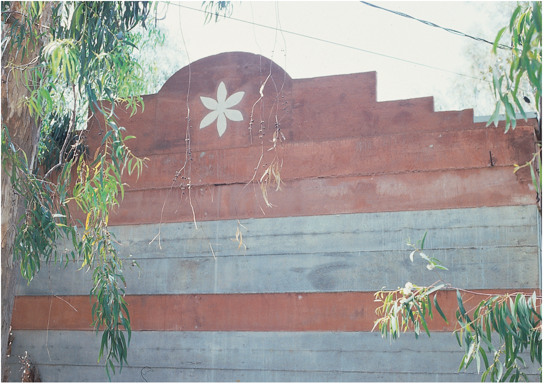
Front wall surface of the Sala house. Precast white terrazo ornament inserted into the poured concrete wall.
