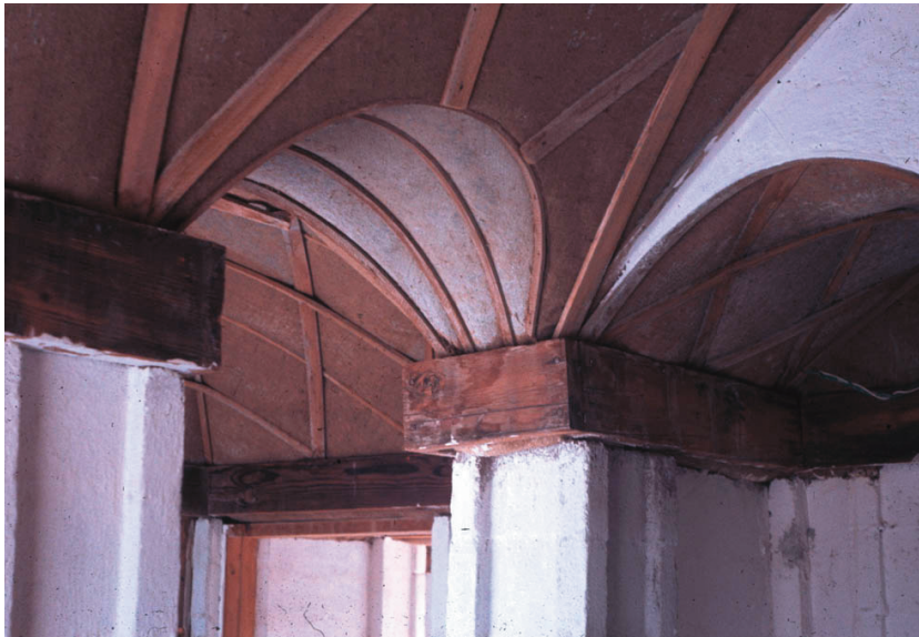
Groin vaults intersection in the lath, burlap, plaster technique of making vaults. Mexicali, 1977.
