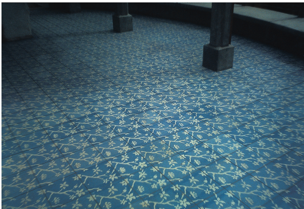
Terrace, Sullivan house, Berkeley, California. The surface of this terrace is made of 800 tiles, cast in blue and white terrazzo, ground and polished. Christopher Alexander, Katalin Bende, 1996.
