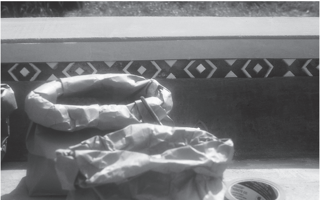
Formwork for an ornamental band on the Fort Mason bench. I thought this ornament was unusually successful—very simple, but satisfying. Christopher Alexander, 1984
