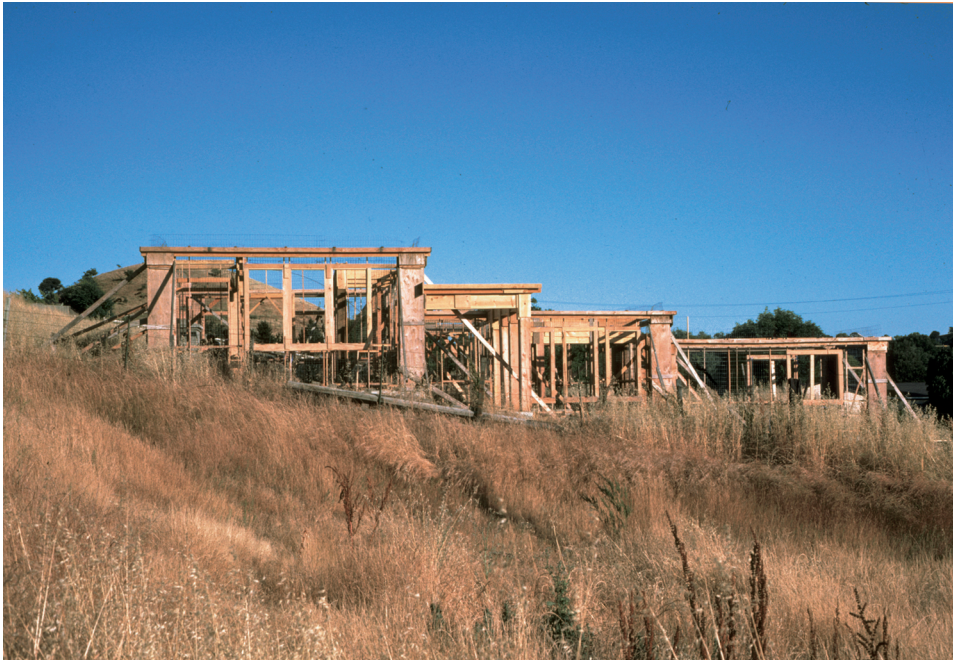
The yellow of the grass—dry, burning—and the light white-blue of the sky. This is a picture of the Martinez house while under construction. You can almost see the color, staring at you, inspiring you, explaining itself to your feeling, even in this photograph. How much more vivid it was, when we were standing there. Christopher Alexander, 1984.
