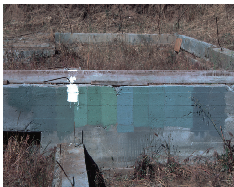
Mixing and testing colors on the Martinez site to get the right wall color.
