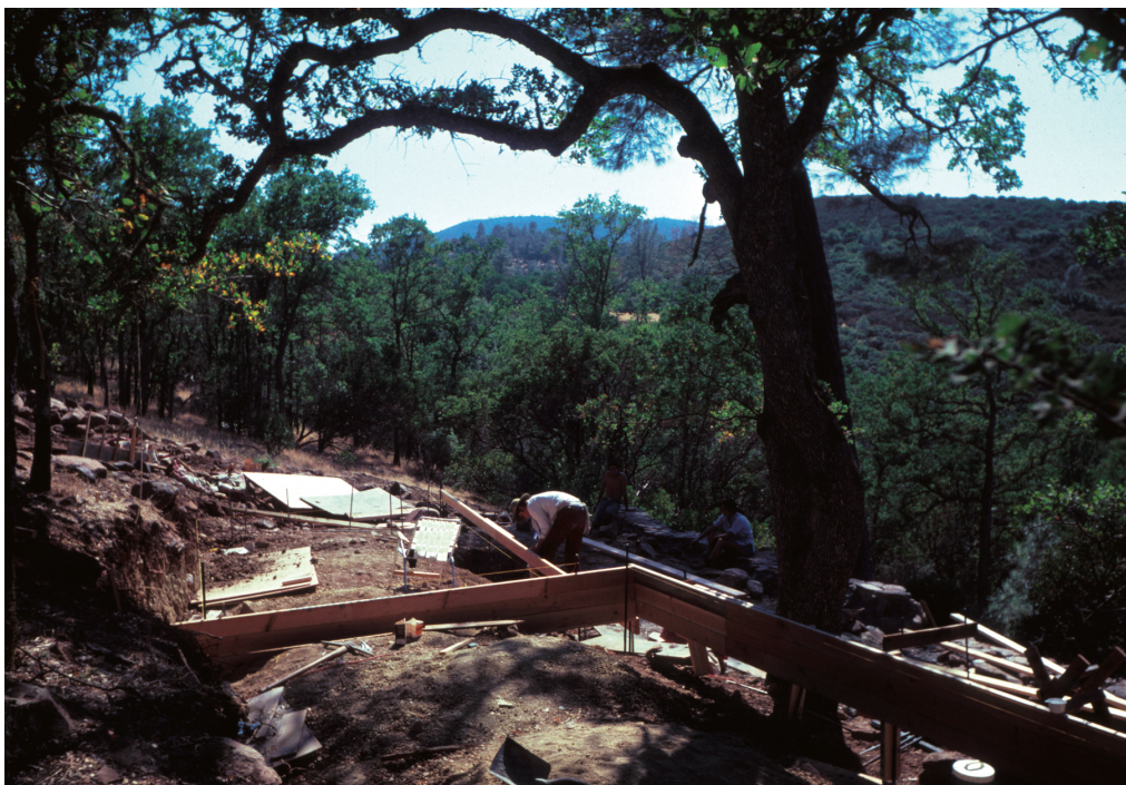
Berryessa house, 1986–87. The site at Berryessa during construction, when both position and design and slab-forming are going on together. Slabs are being placed, carefully, in such a way as to preserve the structure of the land and of the white oak trees. Christopher Alexander with Artemis Aminou and Gary Black.
