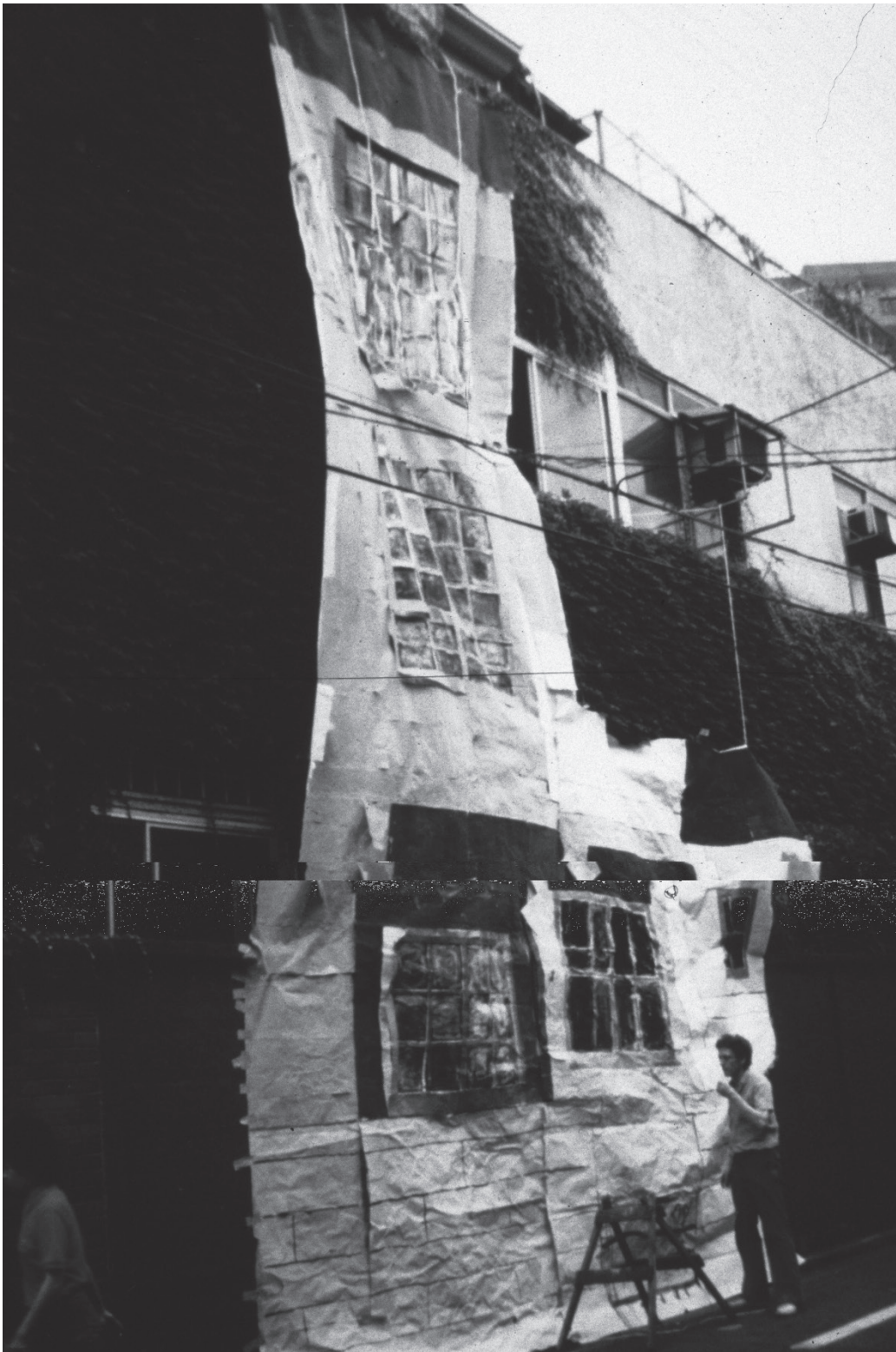
Emoto building, Tokyo. The picture shows Hajo Neis making a fullsize mockup in painted paper on the building that existed previously on the site, to study the effect of the elevation design and materials on the street, so that we could make sure that the street was helped by the building
