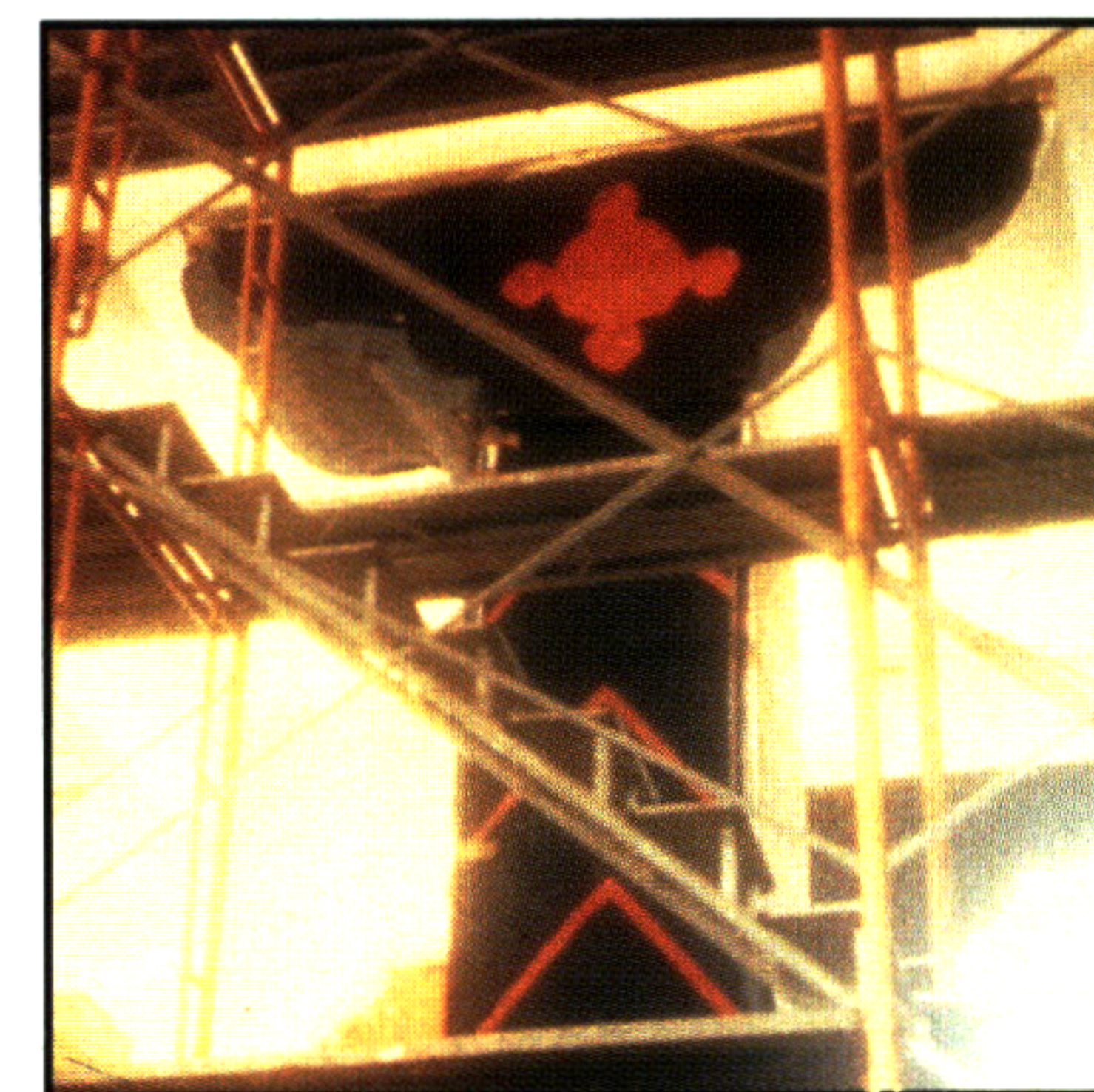
1 . . . . . During construction of the Great Hall at Eishin, huge sheets of paper painted with gouache were hung on the columns (1). When the color and feeling were right, the design was carried out in colored plaster.
