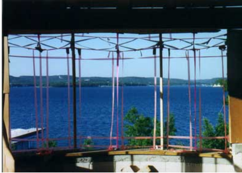
One of perhaps 30 or 40 steps in the use of surveyors tape to visualize the right window.
