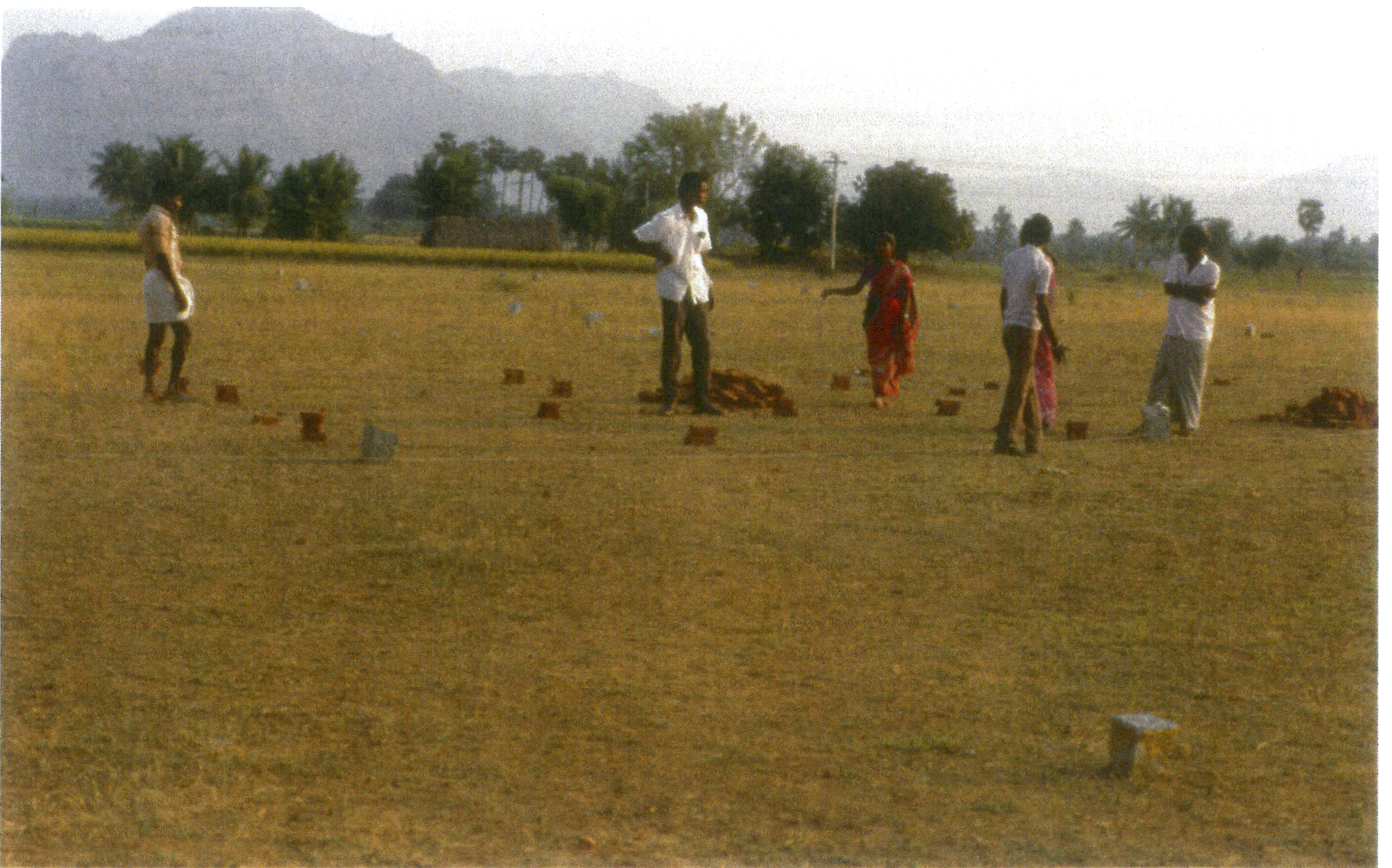
Families of cycle-rickshaw drivers laying out site for their new houses at Abdullapuram, near Vellore, Tamil Nadu, India. Project by ILLAM: Centre for People's Housing-Tamil Nadu and Centre for Development Madras. Photograph by Howard Davis.
