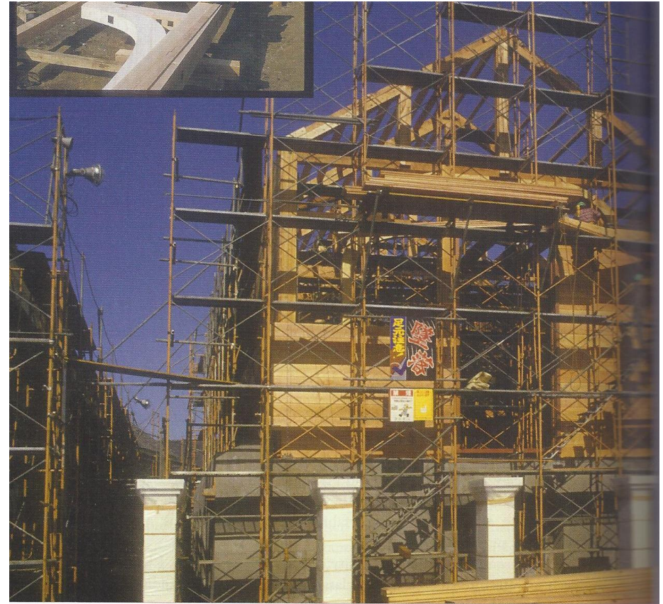
(Page 390) The Central Building under construction in 1984. As we see here, although this building is relatively large, it is being put together in a way of working which allows individual craftsmen to work piecemeal, keeping their individual tasks at their own scale, yet allowing people, cooperatively, to create a relative large and complex whole.
