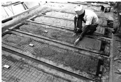
Production of wall panels. Pressed metal and wood frame molds. Casting on floor of house. 1 cm of concrete laid in mold, precut mesh laid over and distance pins with angled bottoms pushed under mesh into wet mix. Final 1 cm of concrete laid over mesh, trowelled around pins and left rough for adhesion of concrete later to be placed in component cavity.
